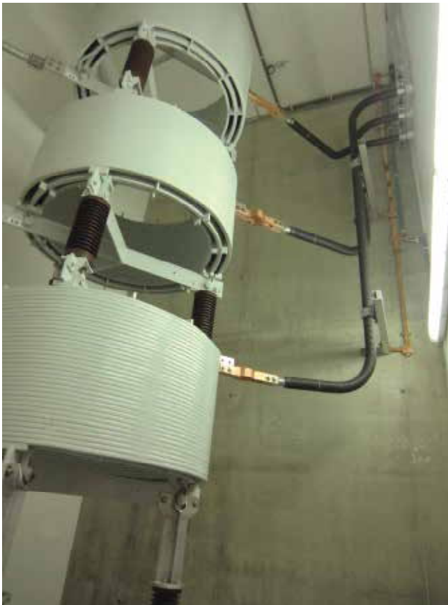
Connection to the current limiting reactors
