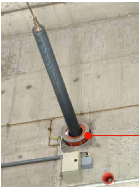
Wall bushing equipped with a current transformer
