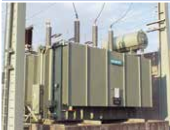
EnBW AG , Siemens Dresden, Germany
