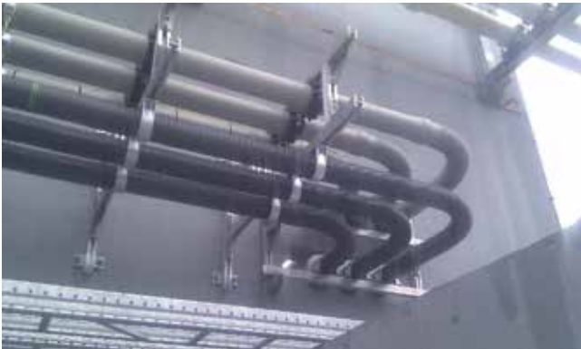
Busbars through the wall
