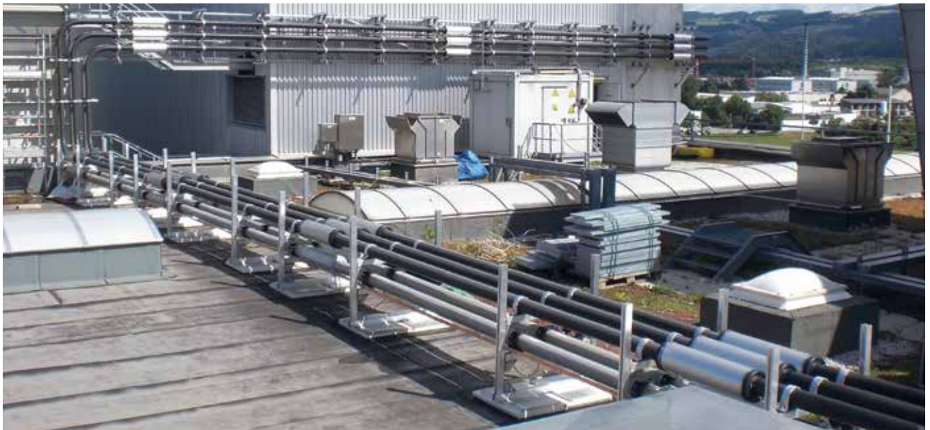
Duresca® busbars in use at the power plant Gud Linz
