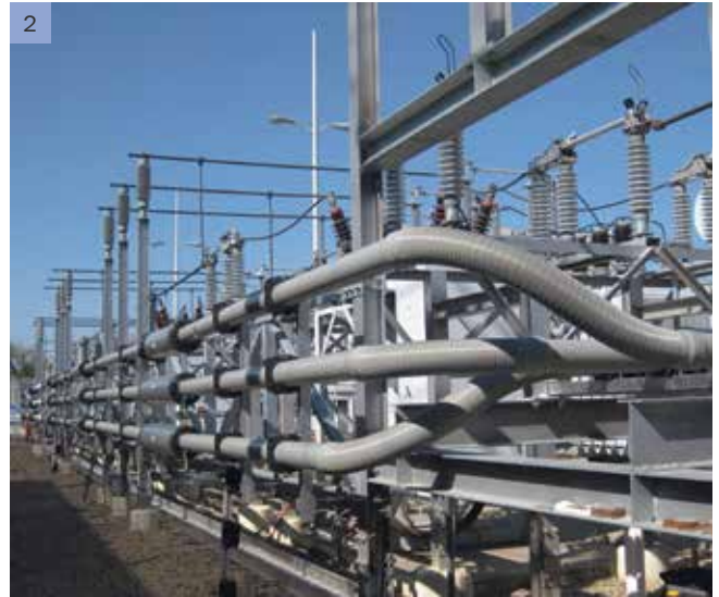
2 72,5 kV EPCOR / Canada (Photo 2) Duresca® in a H.V. application and in outdoor installation.
