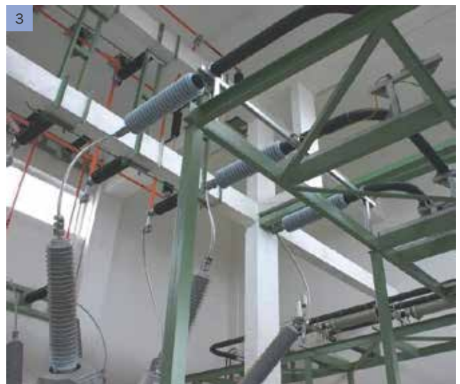
3 110 kV UW Kolin / Czech Republic (Photo 3) Duresca®, the only fully insulated busbar system which is available in the H.V. level, till to 170 kV.
