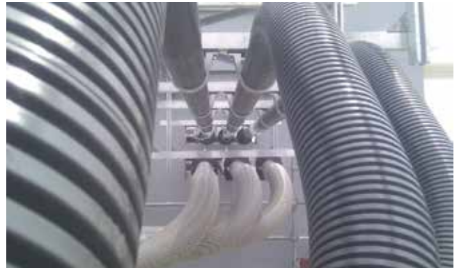
Busbars through the wall
