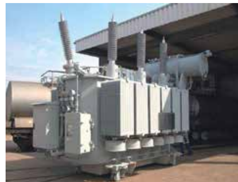
Power Transformer equipped with MGC Bushings
