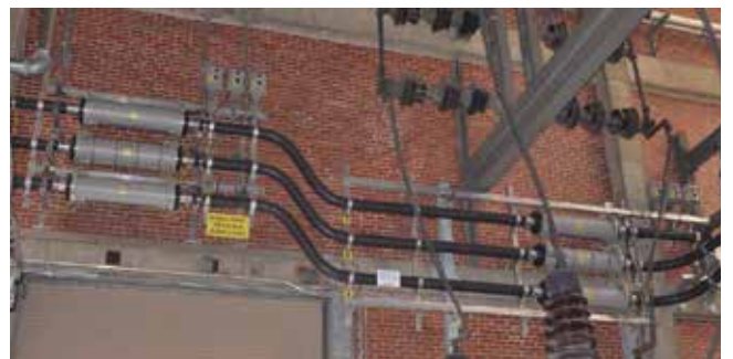
Outgoing line disconnector termination
