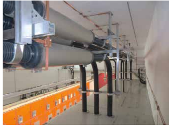
Connection to the switchgears
